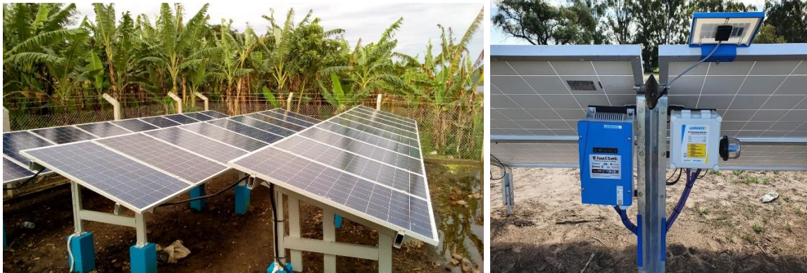
Solar powered water pumping system
